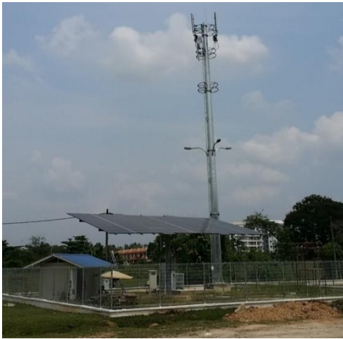
Figure 2. Photograph of tracking PV system for mobile station
