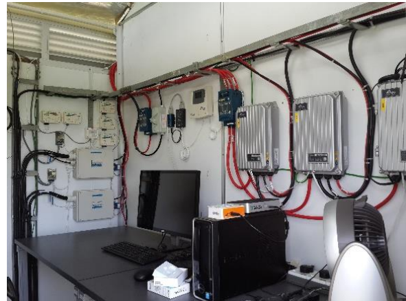
Figure 3. Photograph of charge controller, DC/AC inverter and wireless data logger
