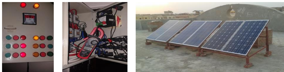
Figure 4. A T S control panel and solar panels
