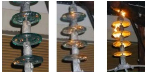
Figure 1. Process of flashover on polluted insulator
