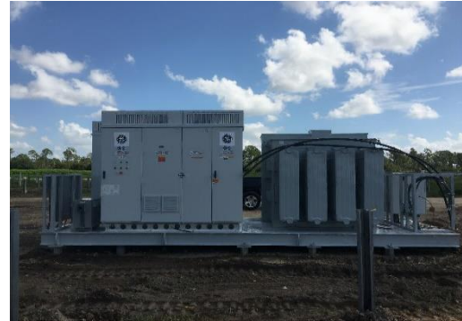
Figure 7: GE's LV5+ SiC-based solar inverter with 99% weighted EU efficiency [46]
