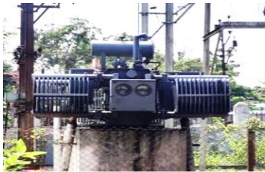
Figure 3. 500 kVA distribution transformer
