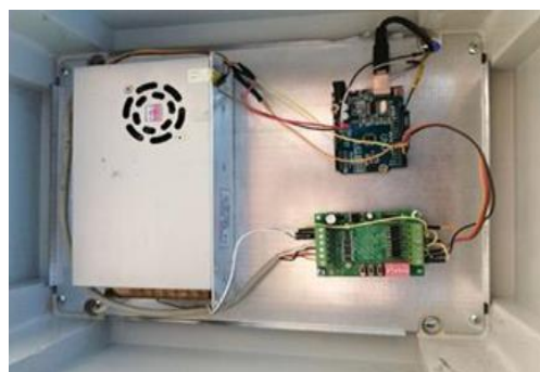
Figure 5. Automated solar collector controller
