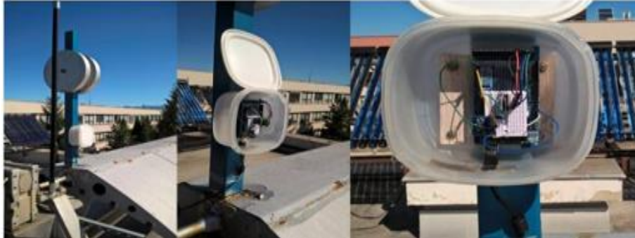
Figure 6. Automated controller with protective housing
