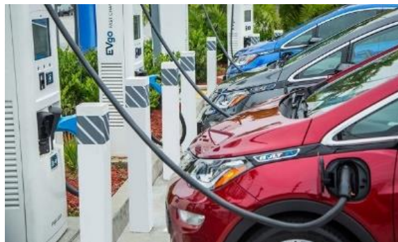
Figure 3. EV charging station
