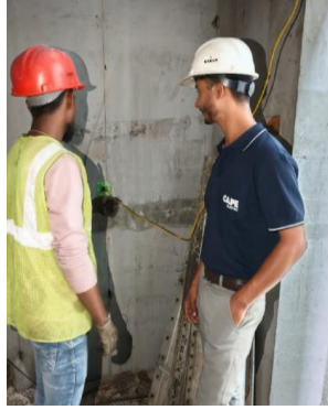
Figure 2. Connection of the earth stud with an MS solid round conductor inside the wall
