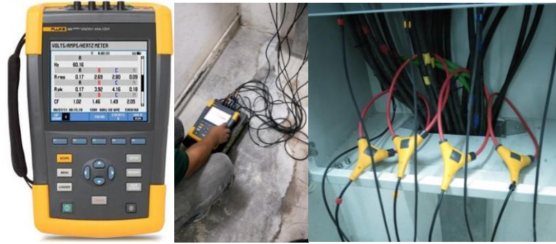
Figure 6. Installation of Fluke 435 PQA for PQ monitoring
