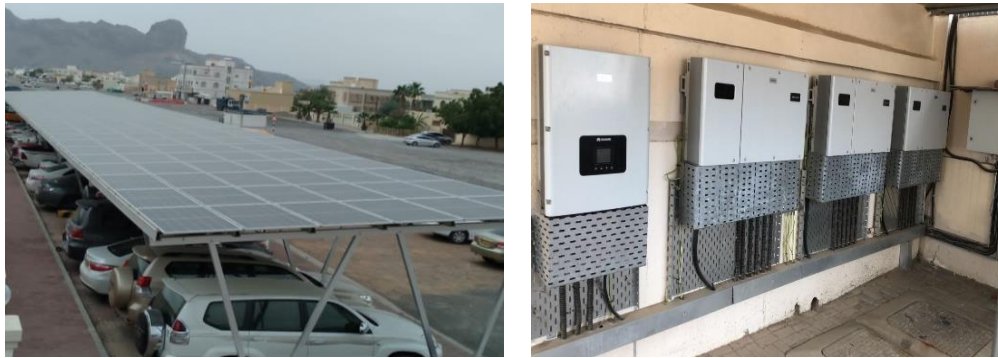
Figure 1. Photos of the 128 kW solar system and the inverter system
