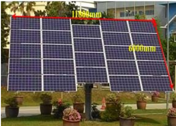
Figure 1. Solar tracking system plant in FKE, UTeM
