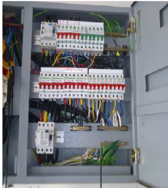
Figure 3. The connection for ground (earthing)
