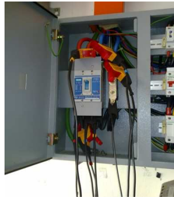
Figure 2 The clamp connection for each phase
