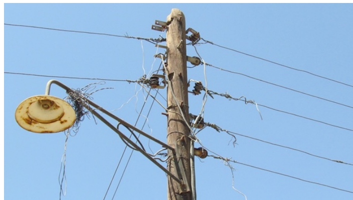
b) The worn existing network (400V) in Isfahan Museum Park
