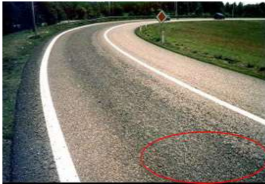
Figure 1. Ravelling in porous asphalt surface layer
