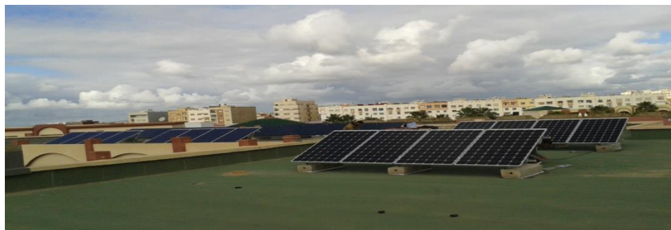
Figure 1. PV Systems Installed in the ESTM
